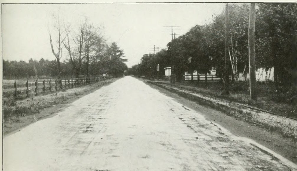
A Bituminous Surface Treatment, State of Massachusetts. Using an oil carrying 70 per cent. of asphalt.
